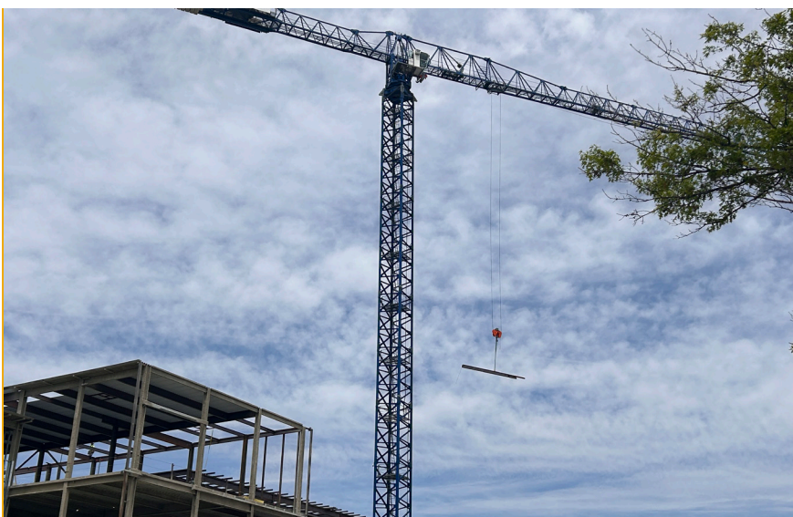
The “Topping Out” Ceremony was Tuesday, April 24. This marked the last steel beam being placed on the structure.
