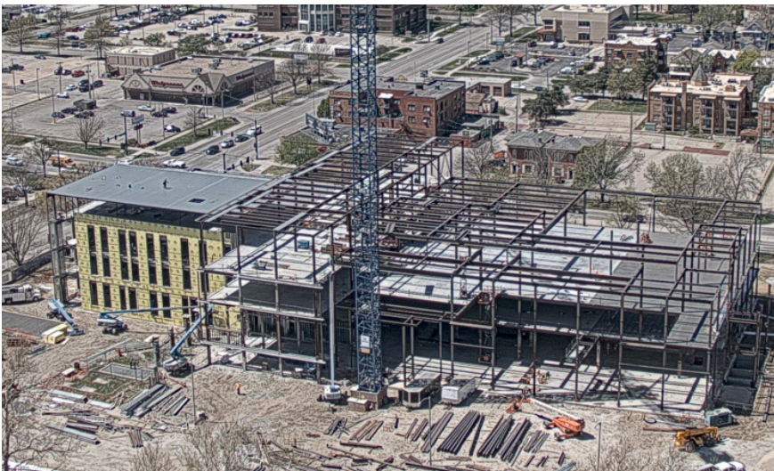
This is the view from the remote camera on April 14. Expected completion is July 2025 so we are just over a year out.
